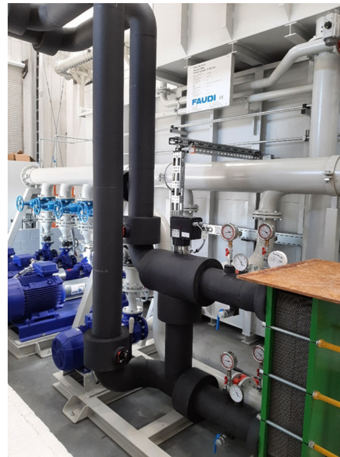
Picture: Insulated piping
